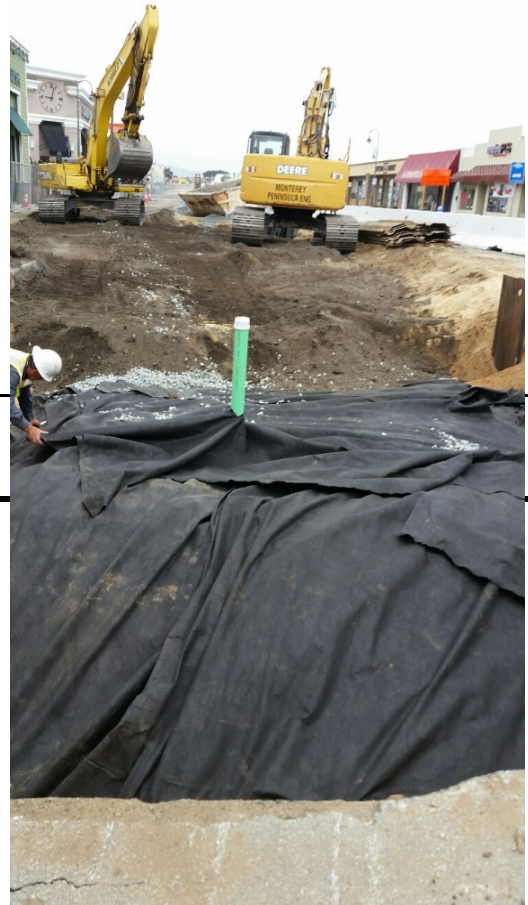
Infiltrator #4 fabric wrap, closed end (east)
