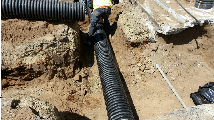
12" HDPE pipe at Drainage Structures 5a and 5c.
