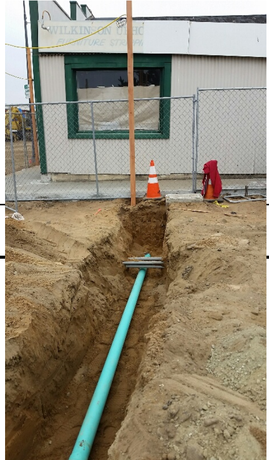
CCO 3 temp lighting sleeve across Hillsdale St
