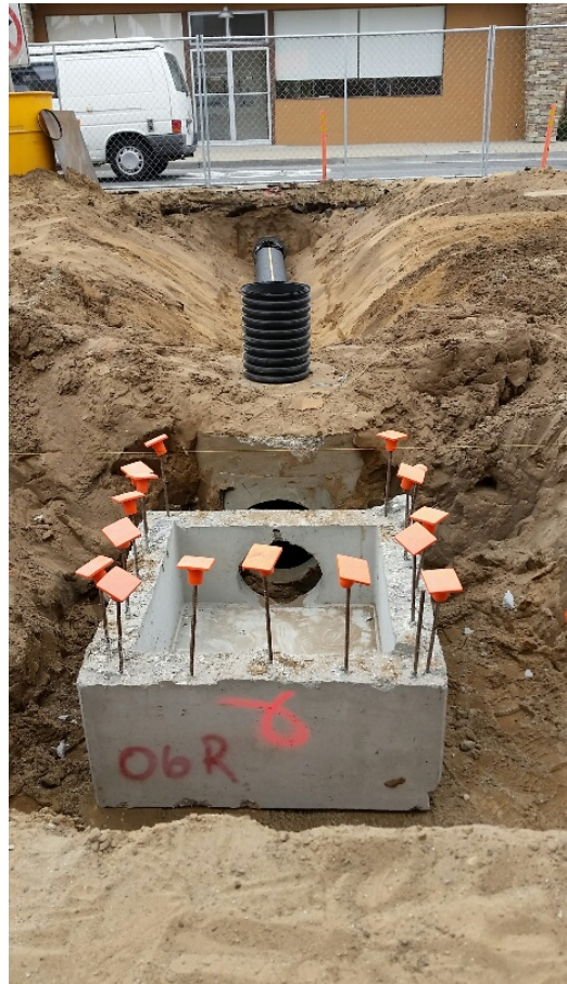
DS 6r (GO inlet) connecting to manhole 6g DS 6u pipe extending to north side of Bway
