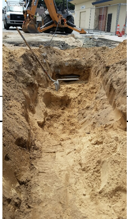
Irrigation and electrical conduit at same elevation as DS 6d
