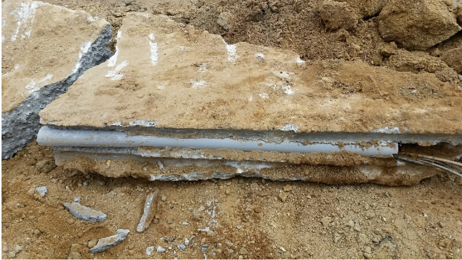
Conduit encased in cement slurry
