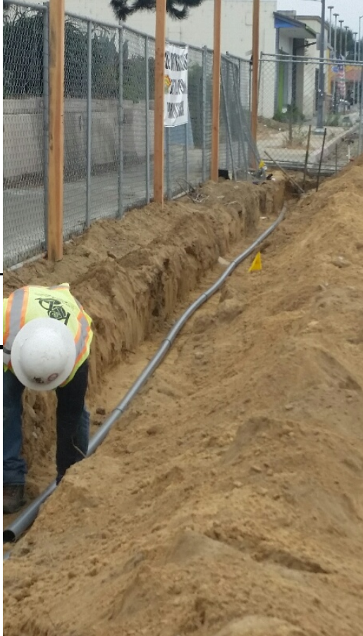
Irrigation trench and electrical conduit, west of Hillsdale St
