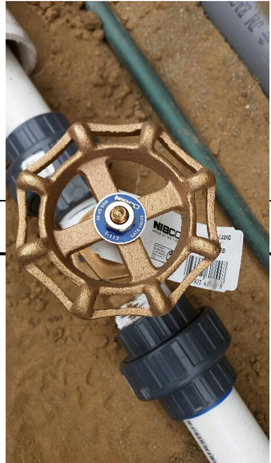
Irrigation gate valve
