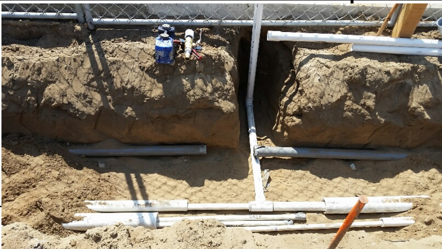
Irrigation connections to bubbler and drip system lines
