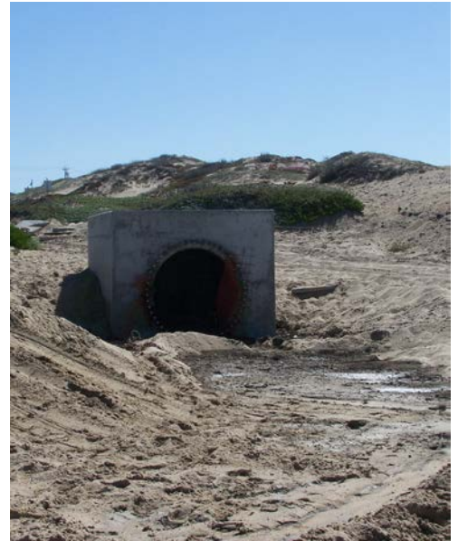
Raised outlet box upstream of the lower Tideflex check valve shown below
