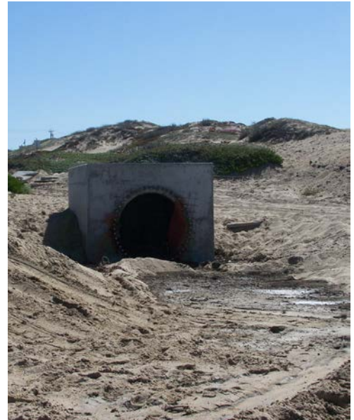
Raised outlet box upstream of the lower Tideflex check valve shown below
