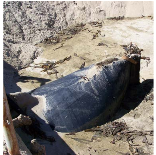
Lower Tideflex check valve blocked by sand
