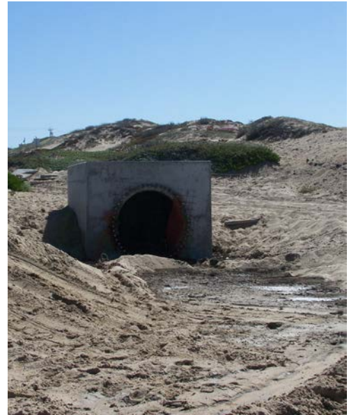
Raised outlet box upstream of the lower Tideflex check valve shown below
